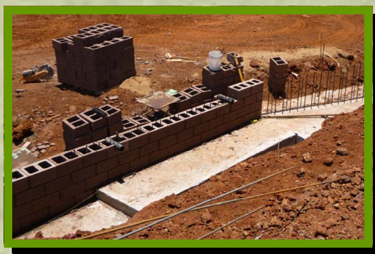
Photo Top - Completion of mass grading and partial construction of the concrete drainage channel. Photo Bottom - Construction of the first lift of the site retaining wall. Each lift was carefully inspected by the structural engineer before proceeding with the next lift.
