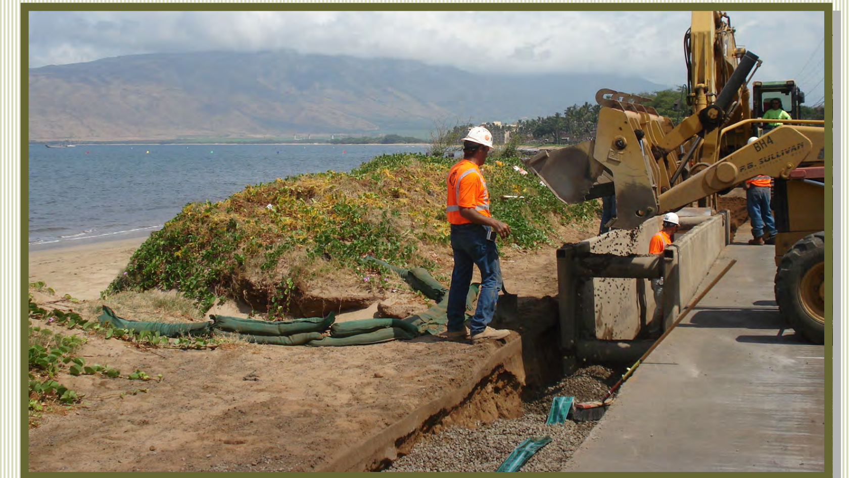
BACKFILLING TRENCH - Pipe being backfilled with tracer tape on top. Special precautionary measures were taken to avoid disturbance to sand dunes.
