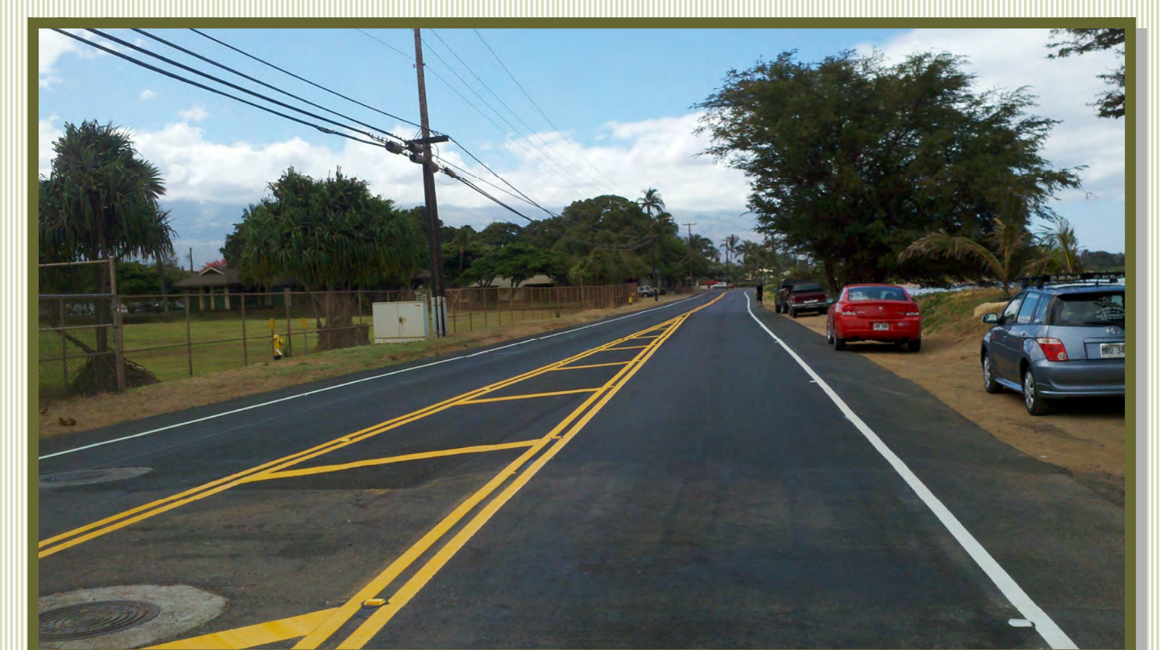
FRESH PAVEMENT - Although the sewerline was only under the makai side of the roadway, the entire roadway width was repaved.
