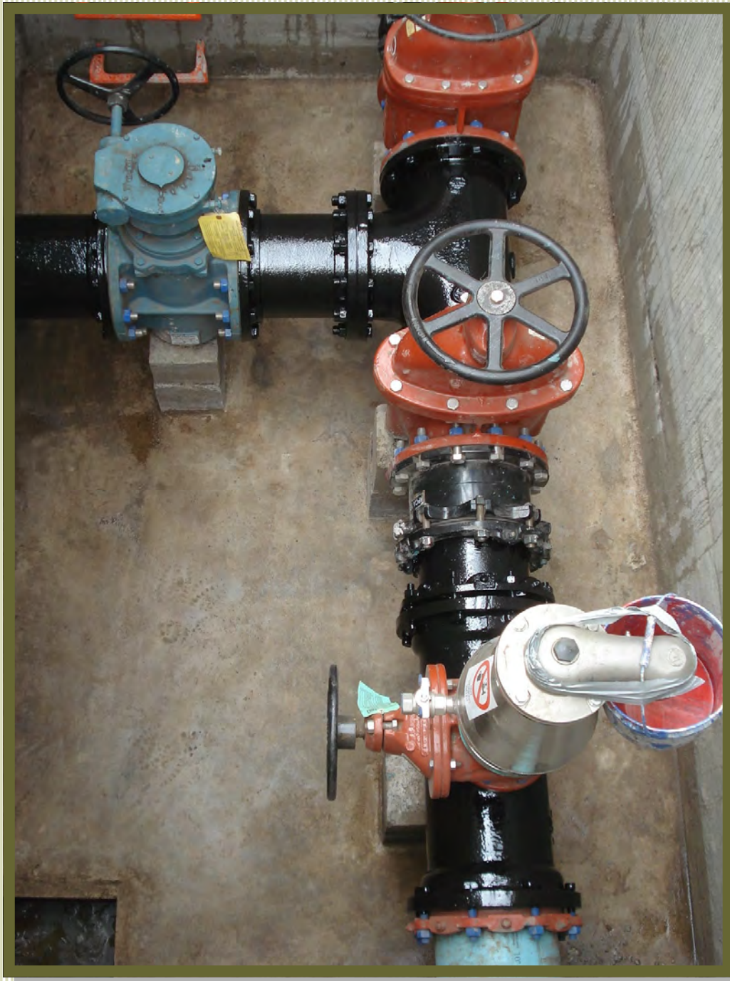
BYPASS VALVE VAULT – Special equipment for wastewater lines. Plug valve on left and air release valve on bottom right.
