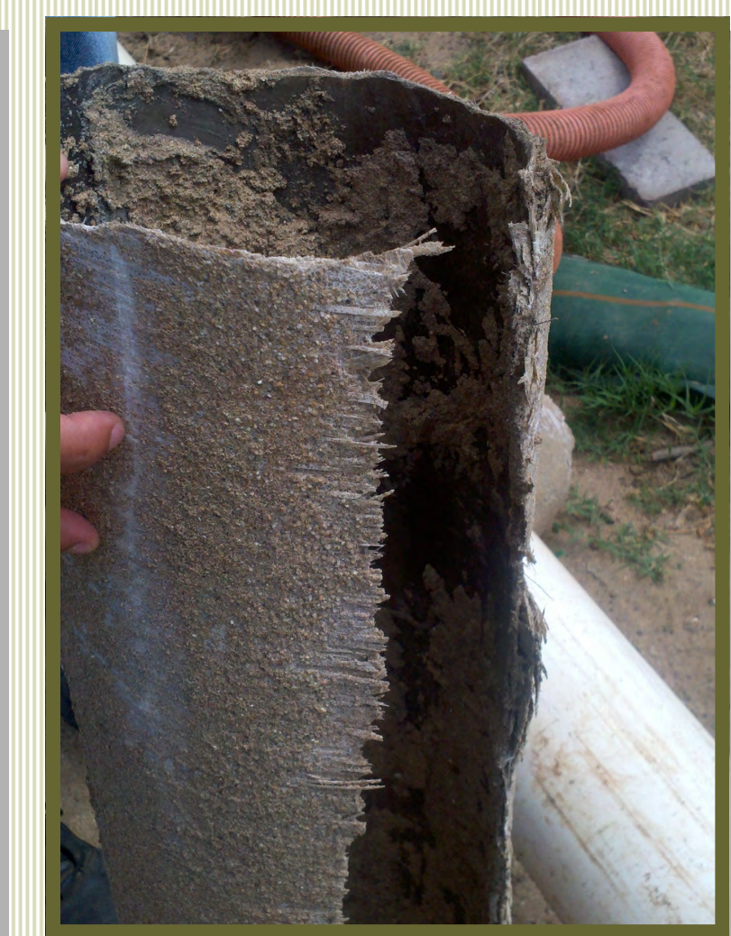
OLD SEWERLINE – Portions of the original sewerline installed in 1975 needed to be removed. The sewerline was abandoned in 1984 because it was made of fiberglass reinforced material with a history of catastrophic failures.
