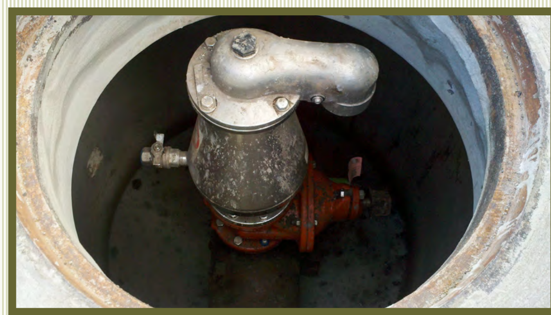
AIR RELEASE VALVE ON SEWERLINE – The valve is actually a combination air valve that allows air to be released from the line, but also allows air to enter if the line empties.
