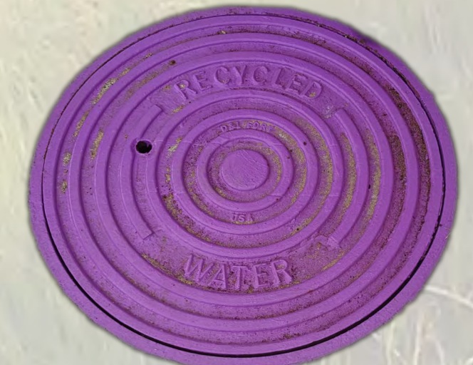
The purple color of pipes, manhole covers, fire hydrants and irrigation sprinkler heads signifies recycled water that is not intended for human consumption.
