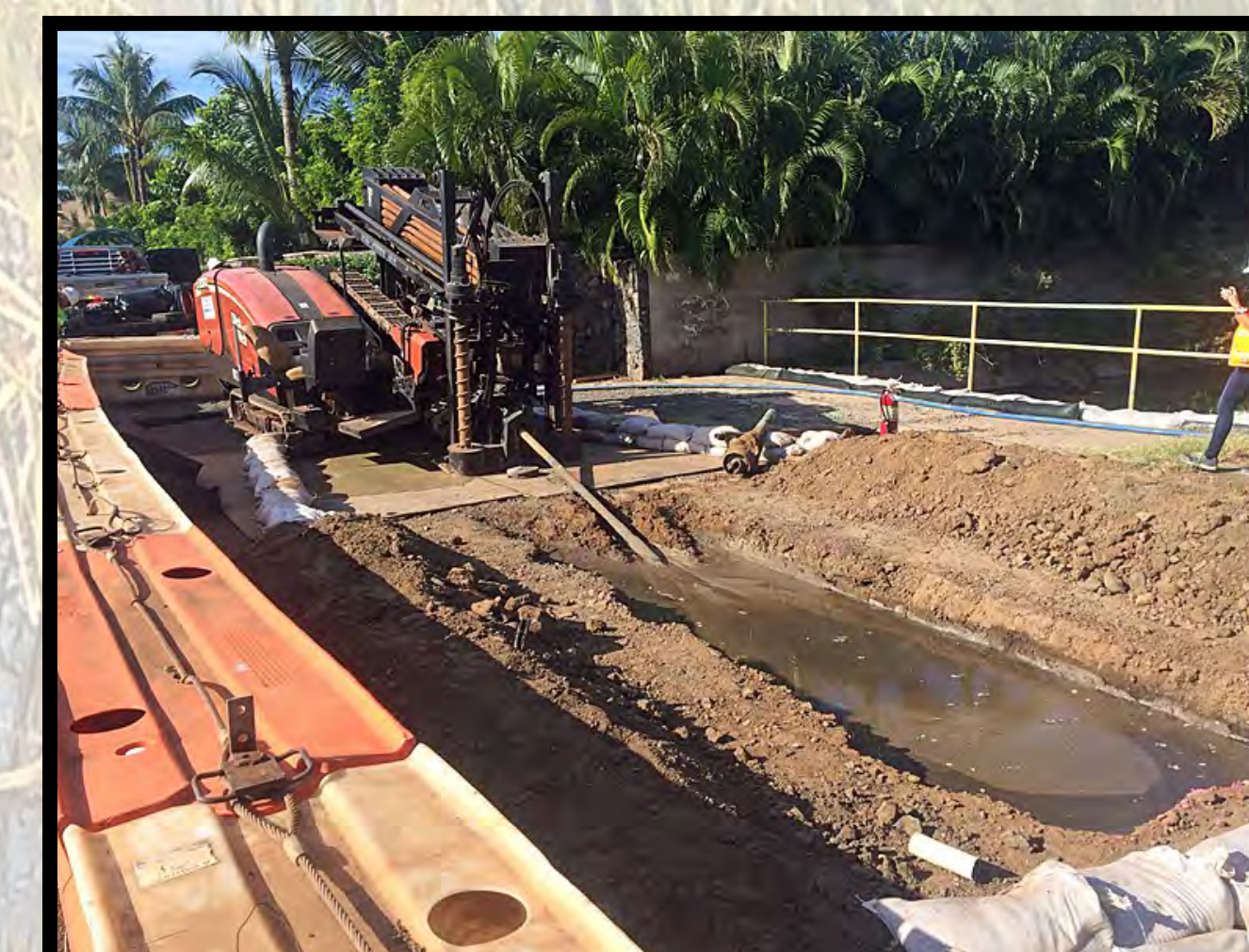
Horizontal directional drilling was used under two drainageways and in South Kihei Road due to: the waterline being installed below the groundwater table, and the need to avoid conflicts with a 36-inch drainline and drainage culvert.
