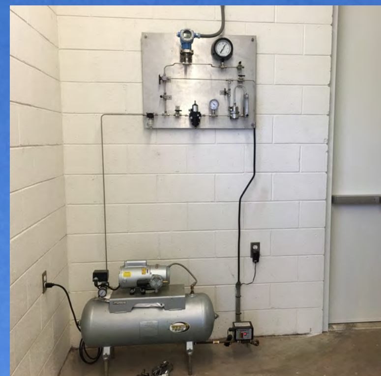
Well level sensing equipment.
