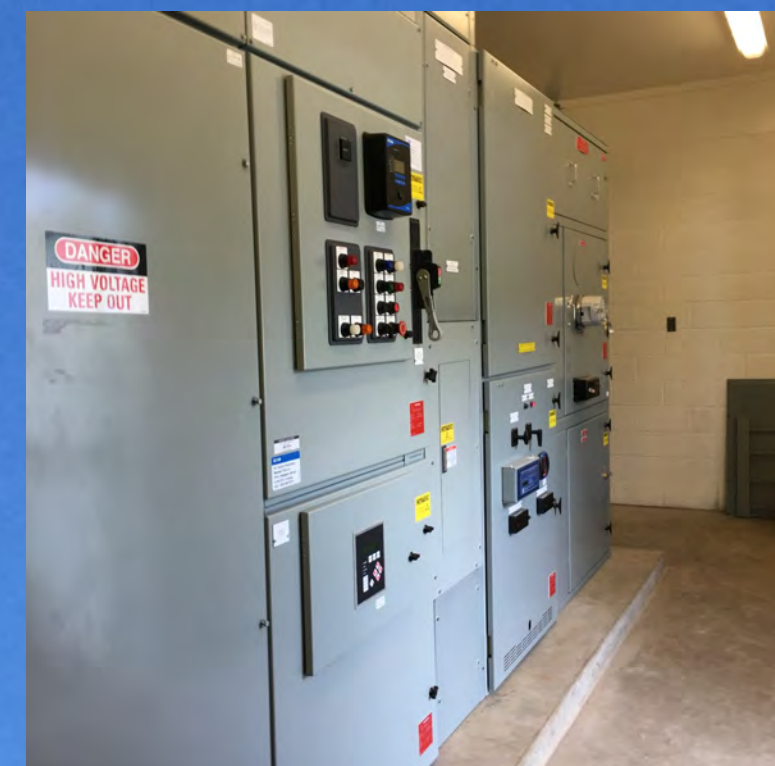
Electrical metering and pump controls.
