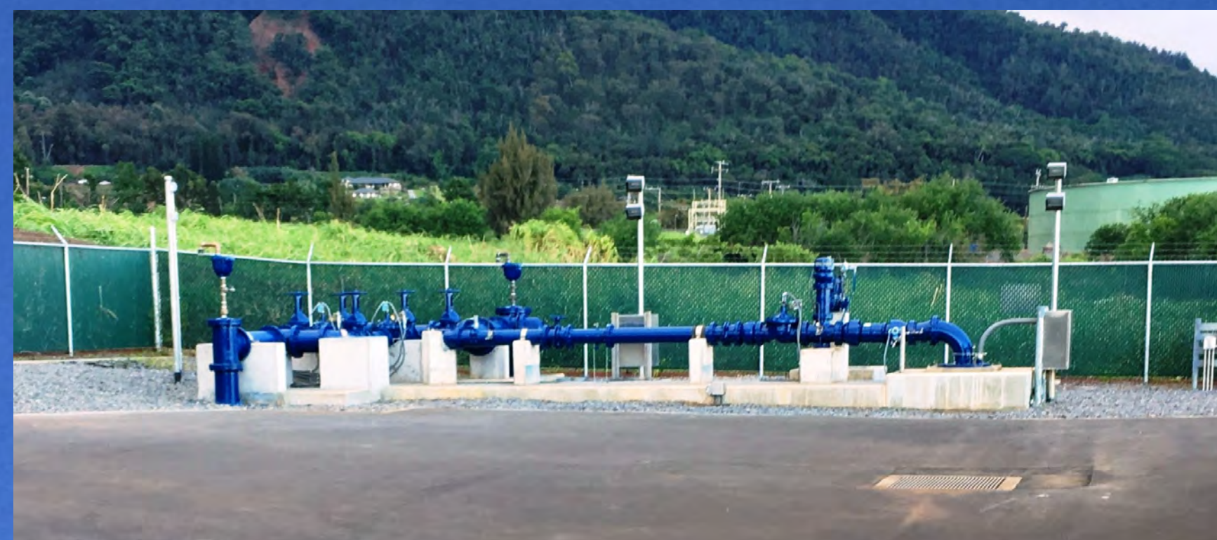
Control valve station for Wailuku Well No. 2 and pump discharge line for Wailuku Well No. 1.
