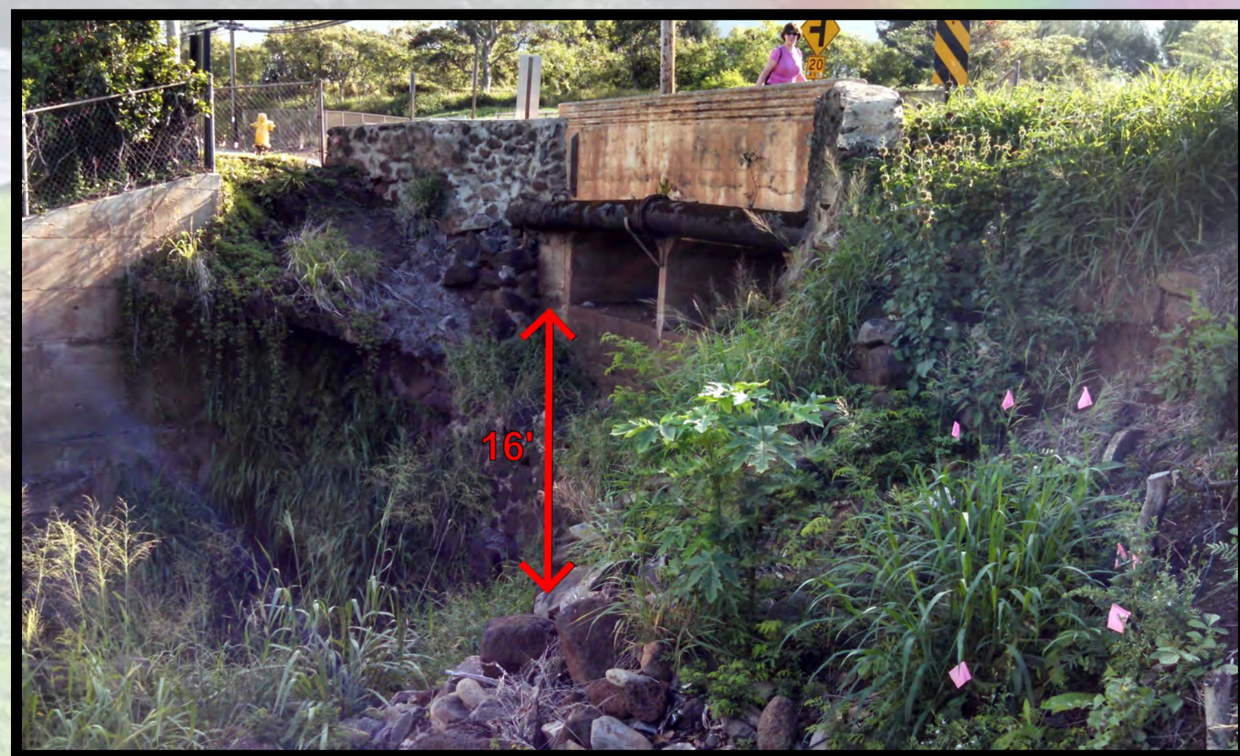
BEFORE: Old, deteriorated drainage structure. 16-foot drop from culverts resulted in flooding on roadway above.
